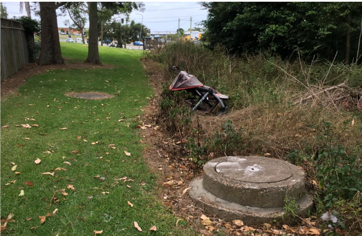
Photo 8: Looking north east towards the Pacific Highway. Rubbish and two stormwater pits are in the foreground
